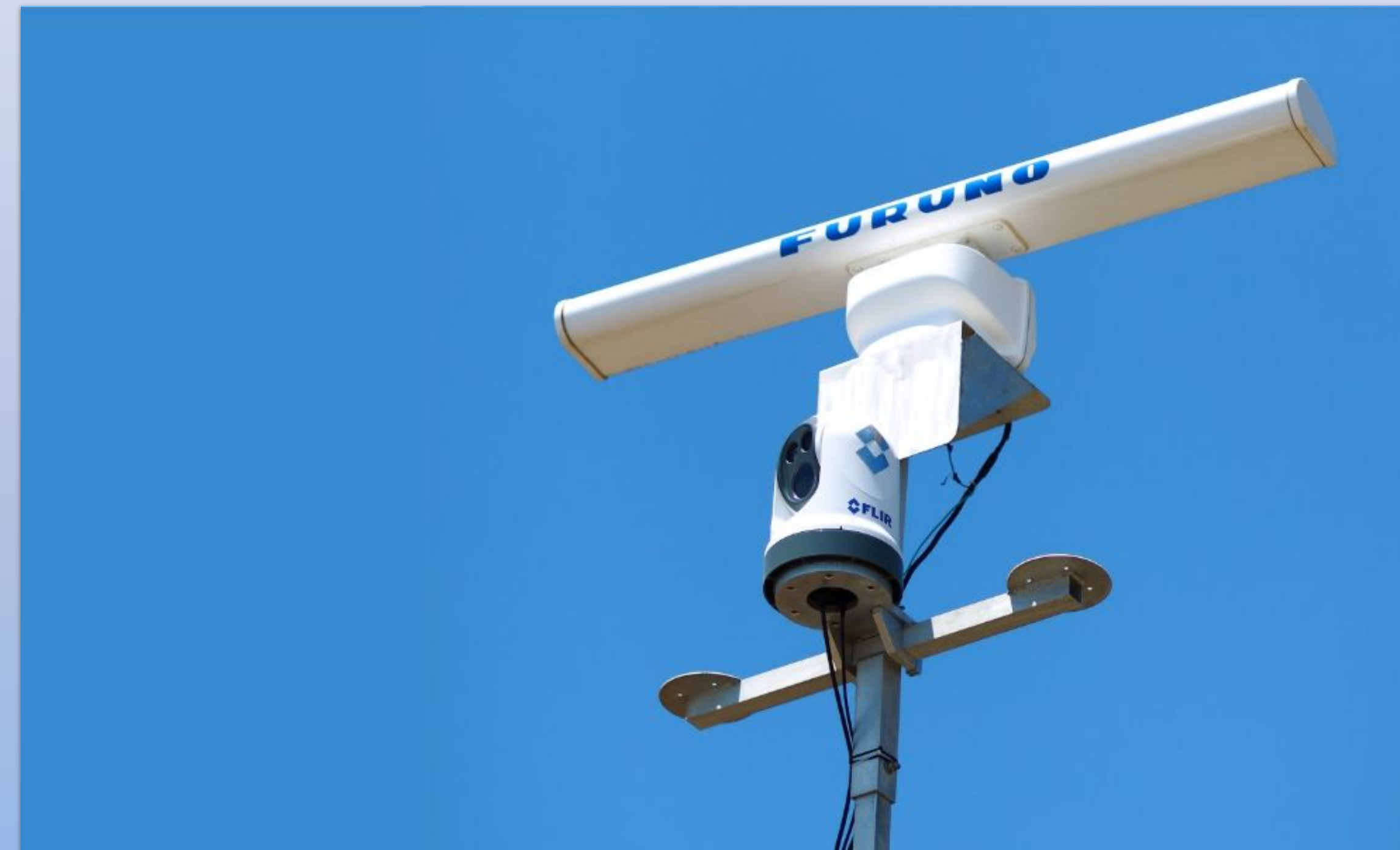
The M400XR installed on the radar tower at Coal Oil Point
